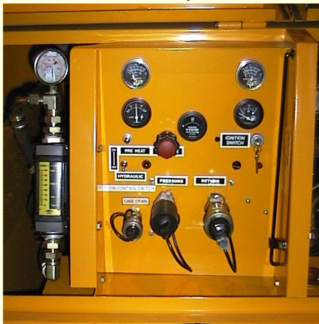
Mod 10 Hydraulic Power Unit Gauge Board
