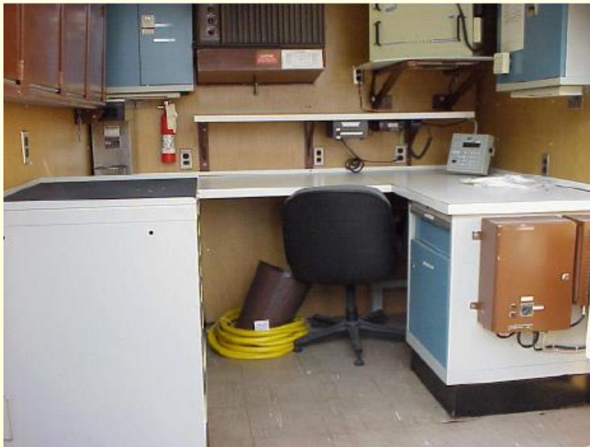
Shipboard Communications System, Van VA0901 Interior
