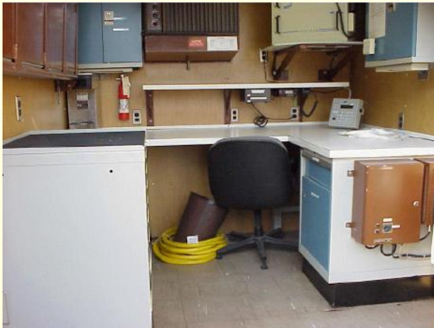
Shipboard Communications System, Van VA0901 Interior
