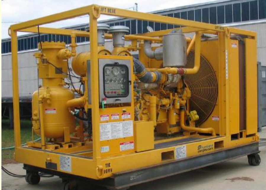
Submarine Salvage Air Compressor AC0245
